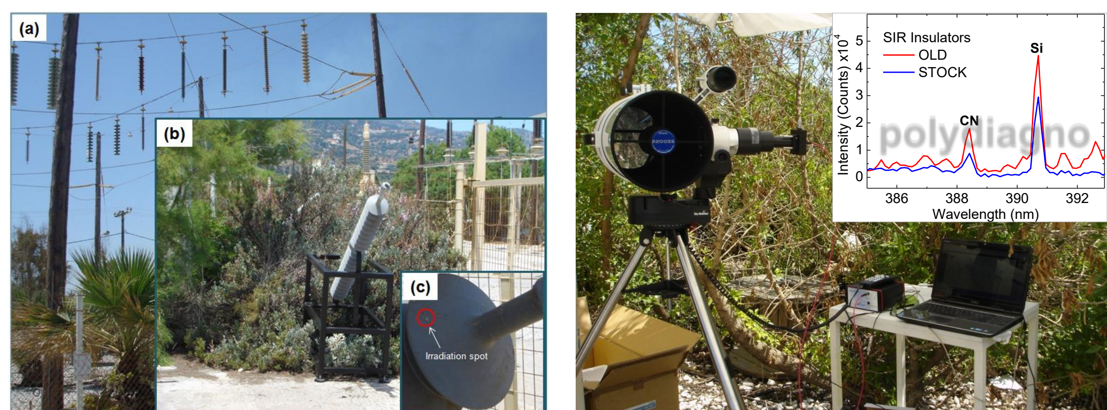
Remote LIBS at the HEDNO High Voltage Tests experimental facility at Linoperamata (Heraklion, Crete)
